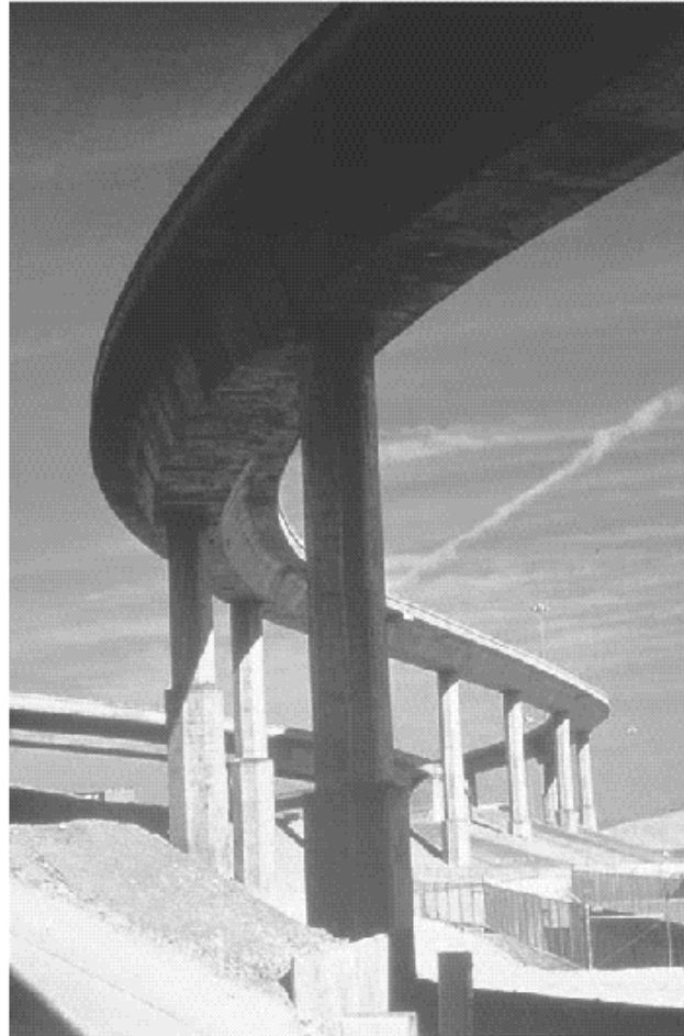
FIGURE 7.2 Curved continuous beam bridge, Las Vegas, Nevada, designed for torsional effects. (Courtesy of Portland Cement Association.)
