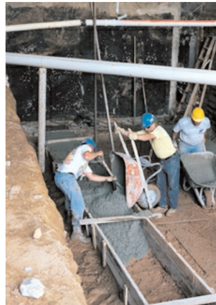
Fig. 11-4. Wheelbarrows are used to place concrete in areas that are not easily accessed by other placement methods. (69929)
