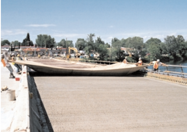
Fig. 11-22. An excellent method of wet curing is to completely cover the surface with wet burlap and keep it continuously wet during the curing period. (69946)
