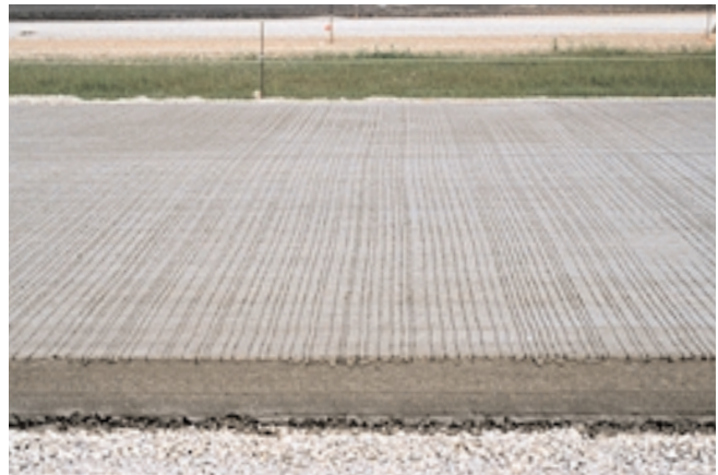
Fig. 11-21. (top) This machine is tining the surface of fresh concrete. (bottom) Tining of pavements improves tire traction and reduces hydroplaning. (69944, 69945)
