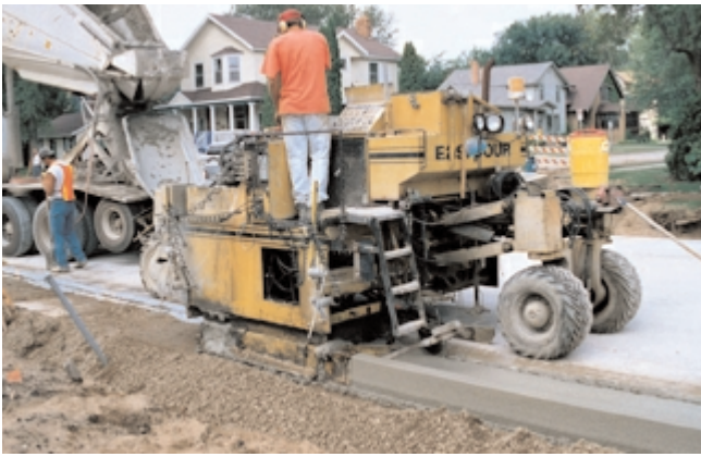
Fig. 11-7. Curb machines continuously extrude low-slump concrete into a shape that immediately stands without support of formwork. (69937)
