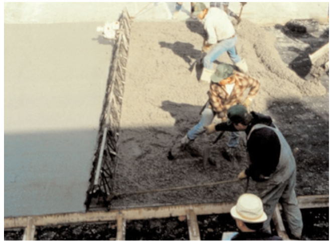
Fig. 11-12. Vibratory screeds such as this truss-type unit reduce the work of strikeoff while consolidating the concrete. (55801)
