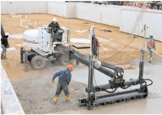
Fig. 11-14. A laser level stimulating the sensors on this screed guides the operator as he strikes off the concrete. Screed poles and chairs are not needed and fewer workers are required to place concrete. Laser screeds interfaced with total station surveying equipment can also strike off sloped concrete surfaces. (69939)
