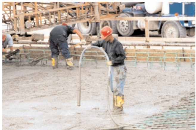
Fig. 11-11. Internal vibrators are commonly used to consolidate concrete in walls, columns, beams, and slabs. (69970)
