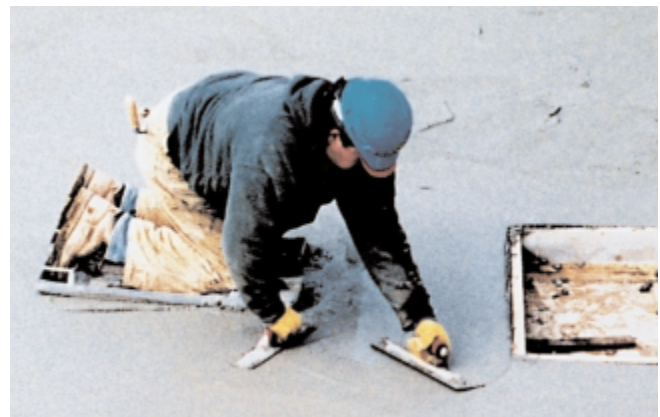
Fig. 11-19. Hand floating (right hand) the surface with a hand float held flat on the concrete surface and moved in a sweeping arc with a slight sawing motion. Troweling (left hand) with blade tilted is performed before moving the kneeboards. (69933)
