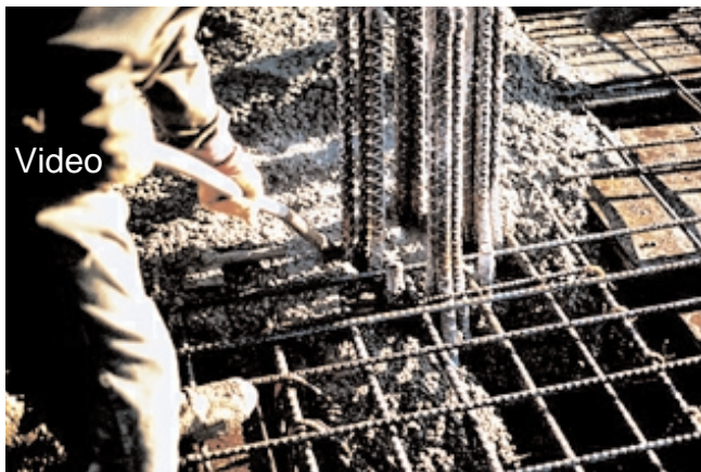
Fig. 11-10. Proper vibration makes possible the placement of stiff concrete mixtures, even in heavily-reinforced concrete members. (55806)
