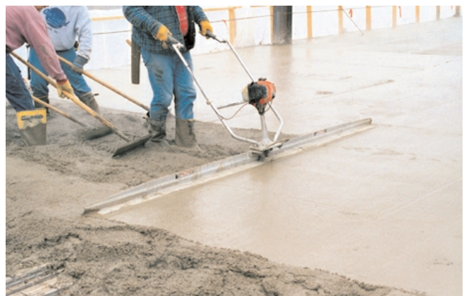
Fig. 11-13. Where floor tolerances are not critical, an experienced operator using this vibratory screed does not need screed poles supported by chairs to guide the screed. Instead, he visually matches elevations to forms or previous passes. The process is called wet screeding. (69938)
