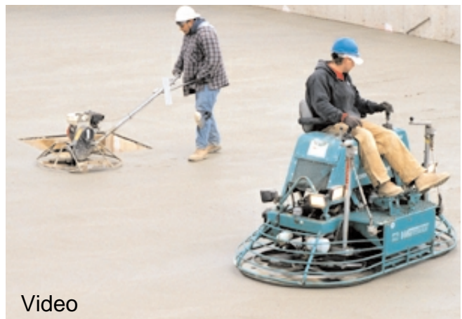
Fig. 11-18. Power floating using walk-behind and ride-on equipment. Footprints indicate proper timing. When the bleedwater sheen has evaporated and the concrete will sustain foot pressure with only slight indentation, the surface is ready for floating and final finishing operations. (69942)
