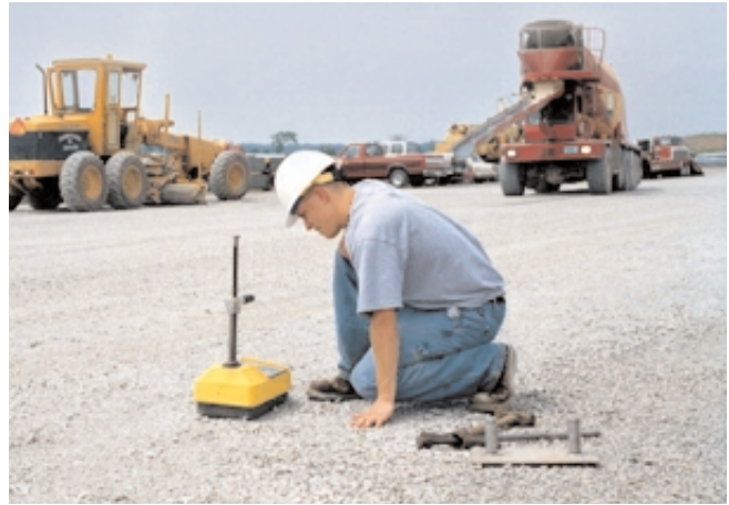
Fig. 11-15. Nuclear gauges containing radioactive sources used to measure soil density and moisture can determine if a subbase has been adequately compacted. (69932)
