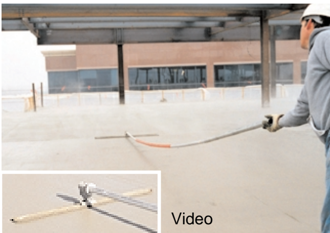
Fig. 11-16. (top) Darbying brings the surface to the specified level and is done in tight places where a bullfloat cannot reach. (bottom) Bullfloating must be completed before any bleed water accumulates on the surface. (70010, 69940, 70011)
