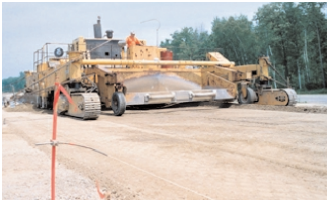
Fig. 11-1. A base course foundation for concrete pavement is shaped by an auto-trimmer to design grades, cross section and alignment by automatic sensors that follow string lines. (69935)
