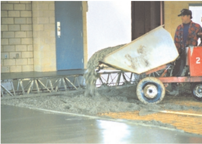
Fig. 11-8. Concrete should be placed as near as possible to its final position. (70009)
