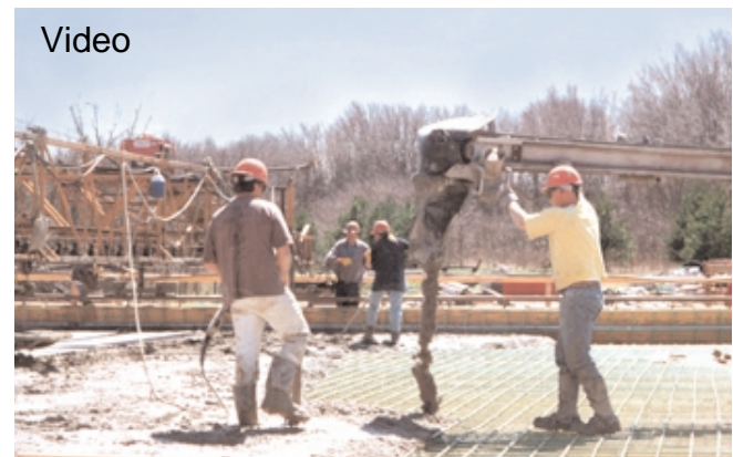
Fig. 11-5. The swing arm on a conveyor belt allows fresh concrete to be placed fairly evenly across a deck. (70002)
