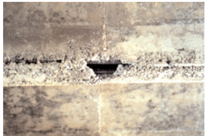
Fig. 11-9. Honeycomb and rock pockets are the results of inadequate consolidation. (50207)
