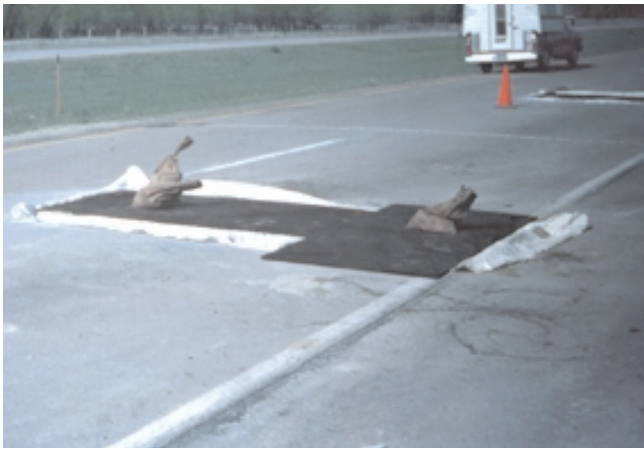
Fig. 11-34. Good curing is essential to successful patching. This patch is covered with polyethylene sheeting plus rigid insulation to retain moisture and heat for rapid hydration and strength gain. (40434)
