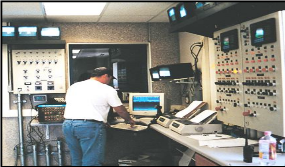
2.1 CONTROL ROOM FOR BATCHING EQUIPMENT IN A READY MIXED CONCRETE PLANT
