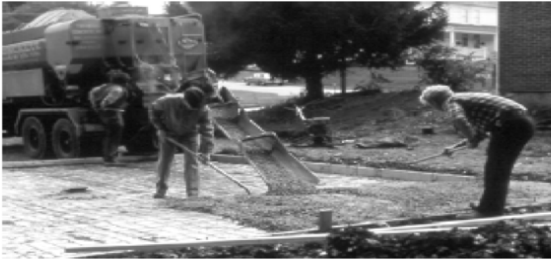
Use of a mobile concrete batching and mixing truck to produce concrete at the job site
